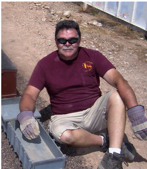
Joe sporting an Arizona Tan takes a short break from track laying*
