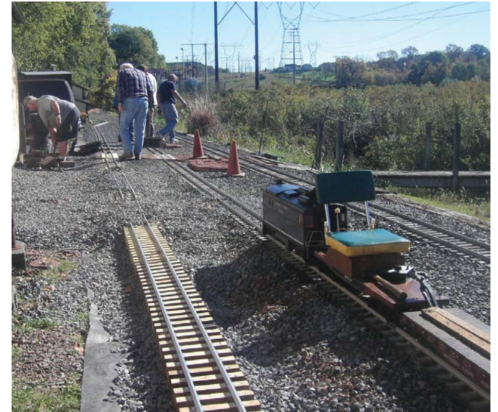
Ballast is applied to the new siding as the work train stands by with the compressor.
